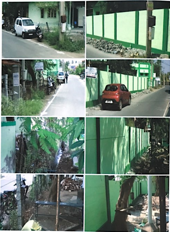
Kovilpalayam PHC Compound wall (Before & After)
